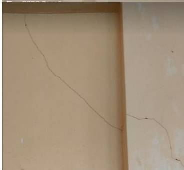
Corner cracks Shear Cracks
