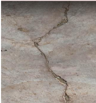
Settlement cracks Shrinkage cracks
