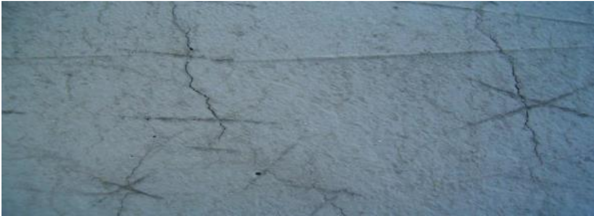
Fig 12: Drying shrinkage cracks
