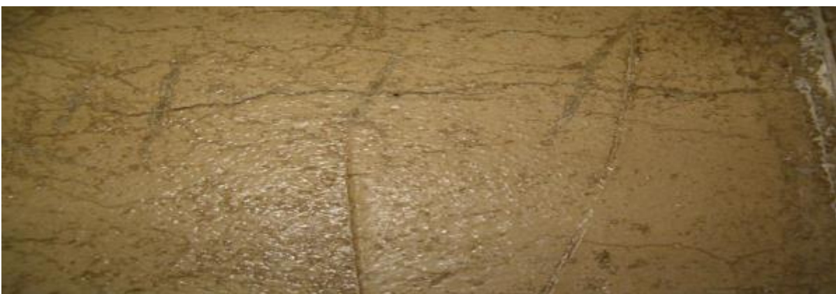
Fig 11: Plastic shrinkage crack
