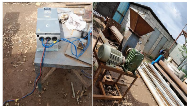
Fig A.3: VFD with complete assembled dewatering machine
