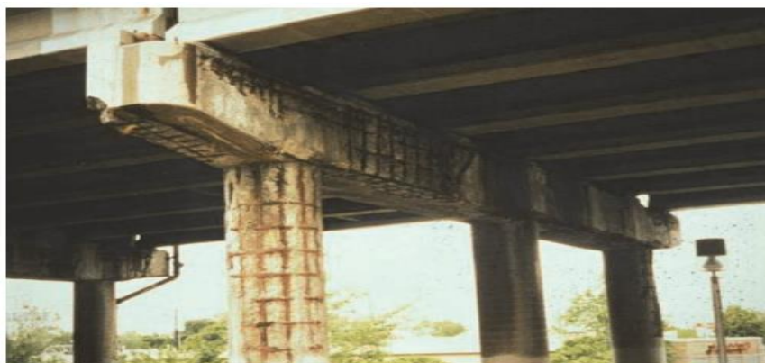
Figure 1.6. Cement reinforced metal piers with corrosion issues [7].
