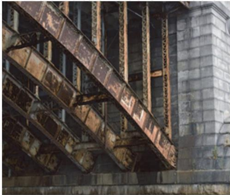
Figure 1.7. Corrosion issues on a structural steel bridge [8].
