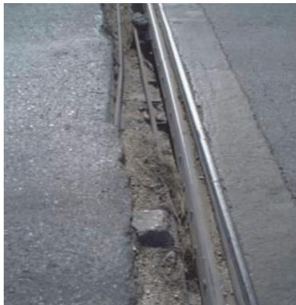
Figure 1.8. bridge concrete construction joint Cracked [9].
