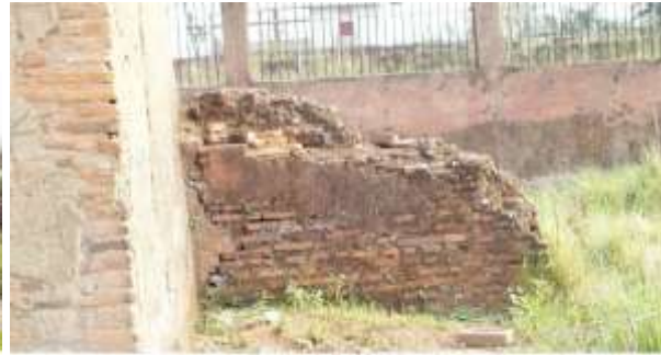
Part of boundary wall of the Ghanashyam Dol
