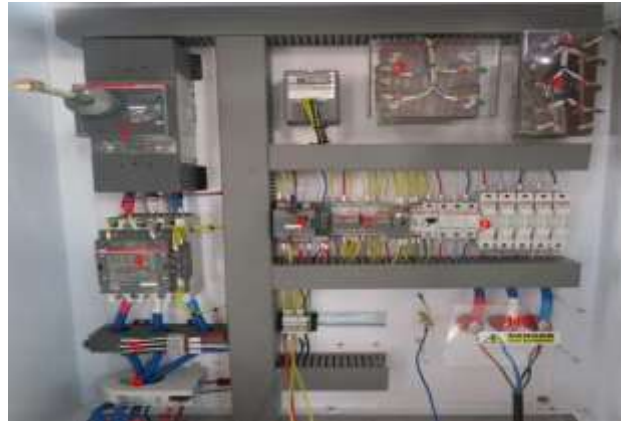
Figure 2: fan control panel
