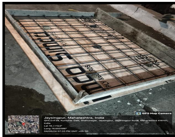
Casting of slab – Use 8mm bar as main bar and 6mm bar as distribution bar
