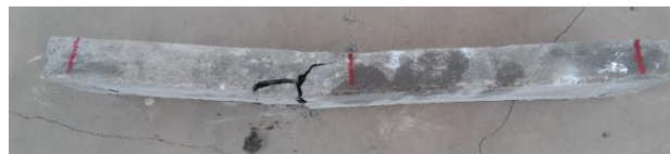
c. Flexure Failure
